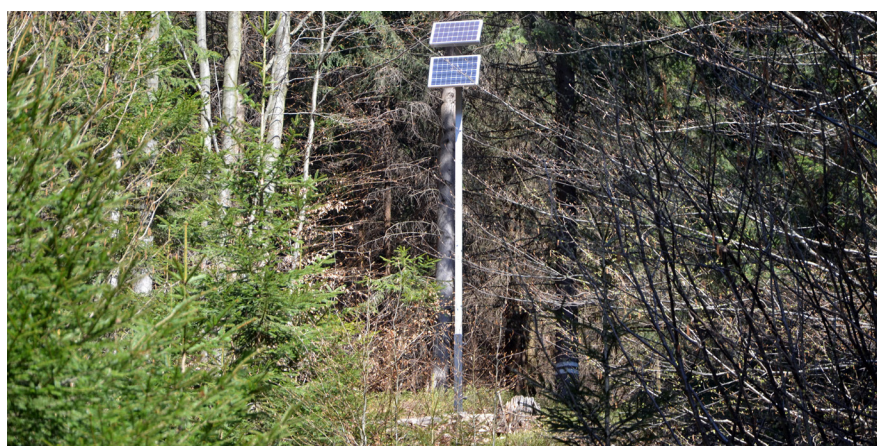
Solar panels that supply the datalogger through battery
